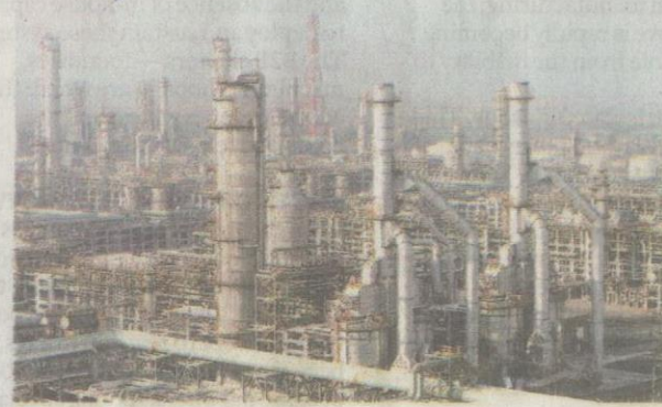
OUTPUT DISRUPTION. Planned maintenance at Reliance's Jamnagar complex significantly reduced exports in May
